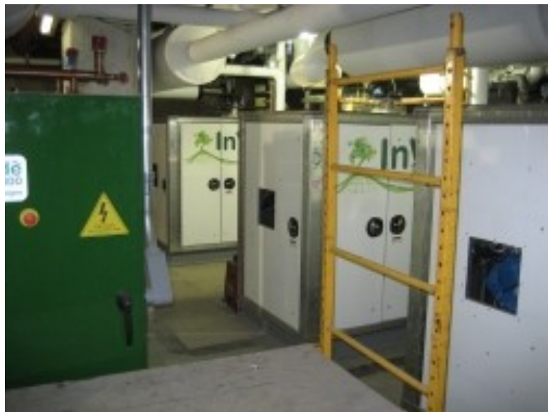
The Brevoort CHP plant consists of four 100kW Tecogen InVerde units which provide heating, domestic hot water and electricity for the 20 story co-op condo building.
