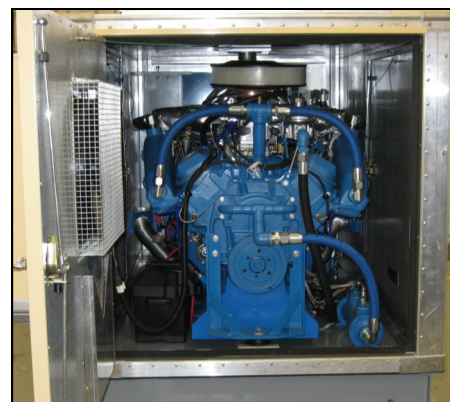
The cogen module is shown inside the weatherproof enclosure pictured in the photo above.
