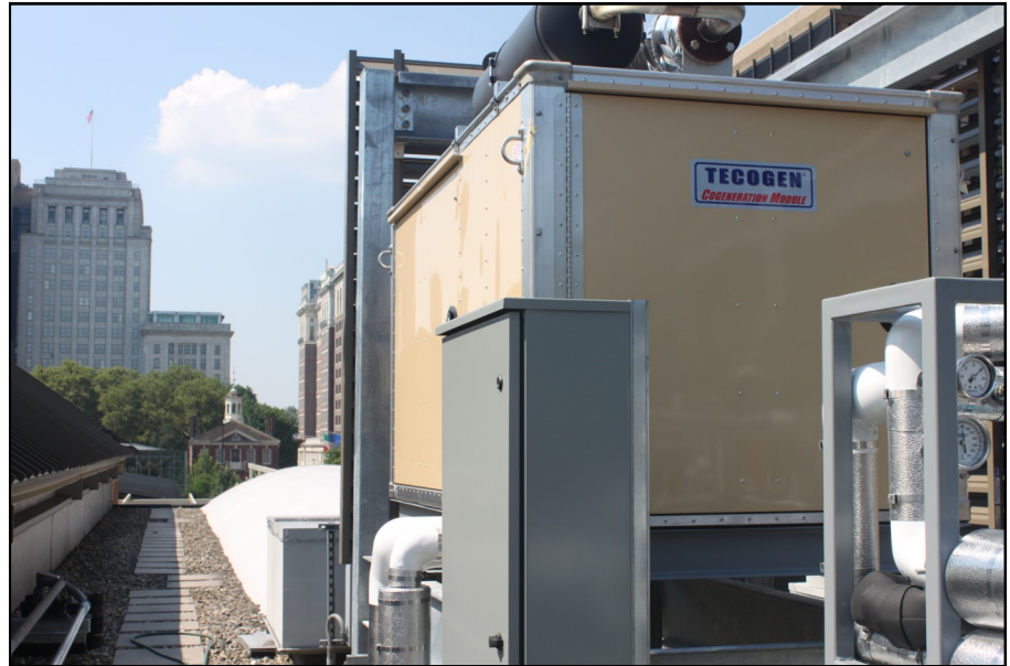
The Tecogen CM-75 cogen module on the roof of the Independence Visitor Center with Philadelphia's Independence Hall in the background.
