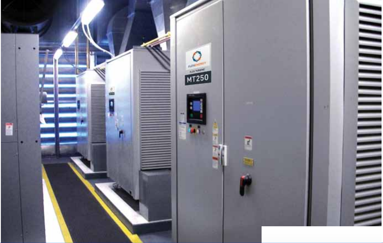
Three 250 kW gas turbines provide both electric power and water heating at the John Muir Medical Center in Walnut Grove, California. Photo courtesy FlexEnergy.
